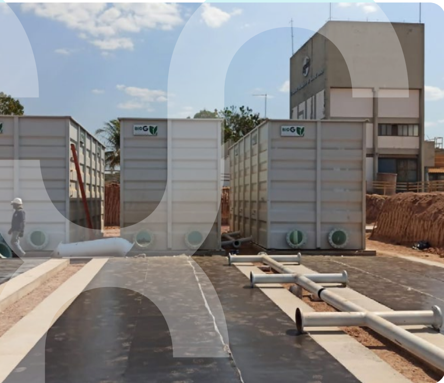
Uruaçu Compact WTP
