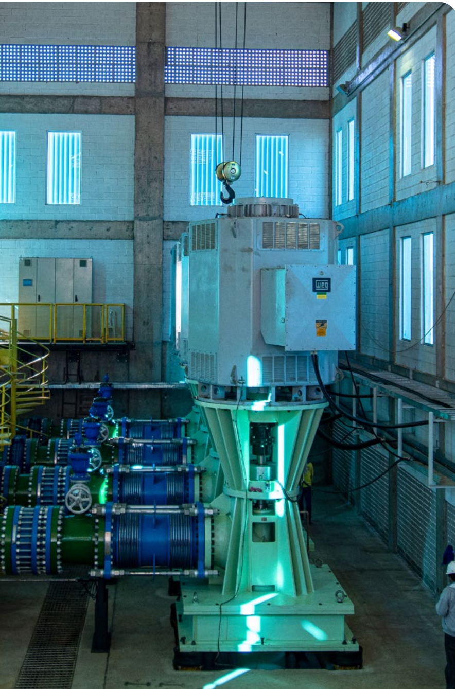
Corumbá System Lift Station
