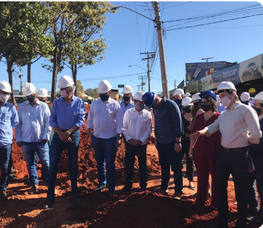
Uruaçu Compact WTP
