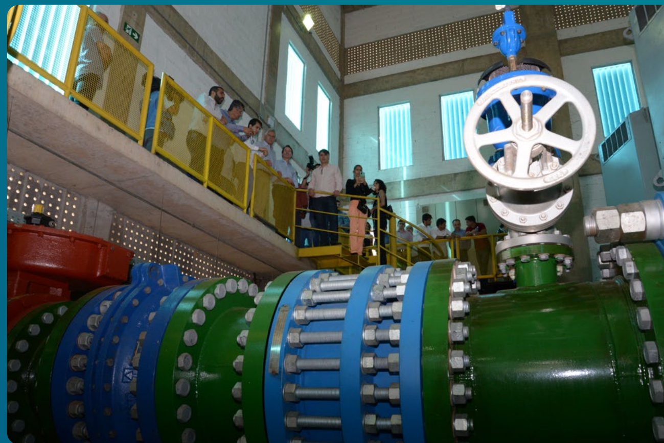
Corumbá System - Saneago Collection
